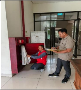
Pengecekan Hydran Berkala
